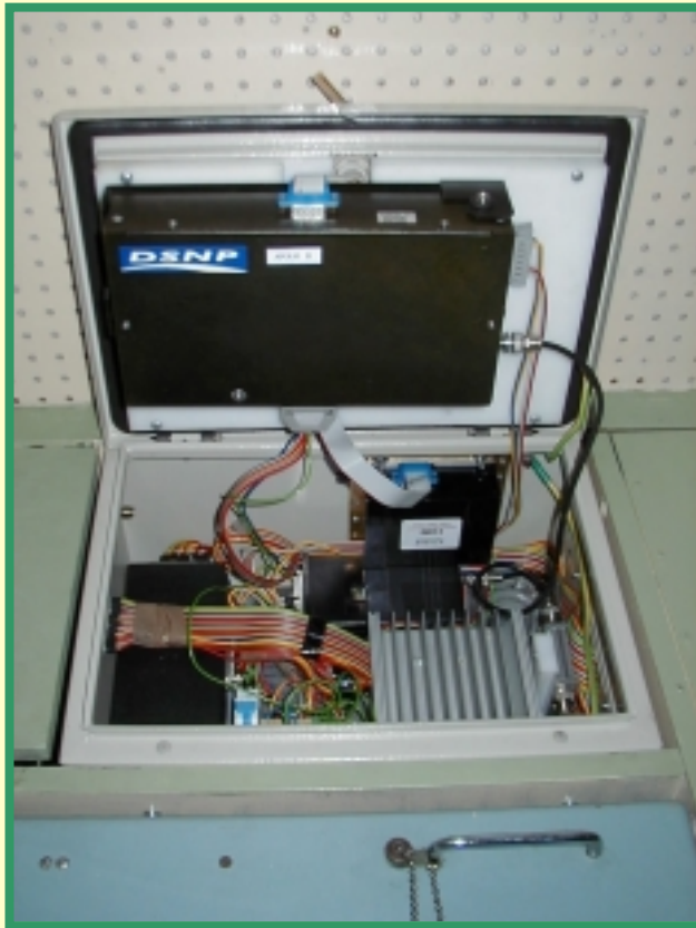
The APOLO train position locator installed on the 130 023-5 electric locomotive.
